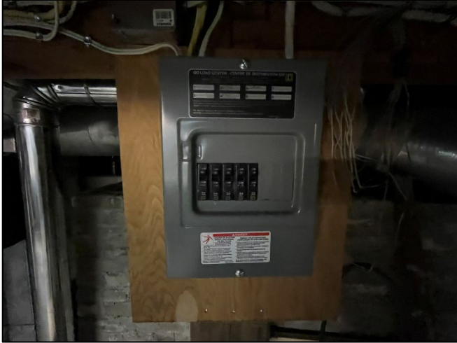
BASEMENT MECHANICS VIEW 3
