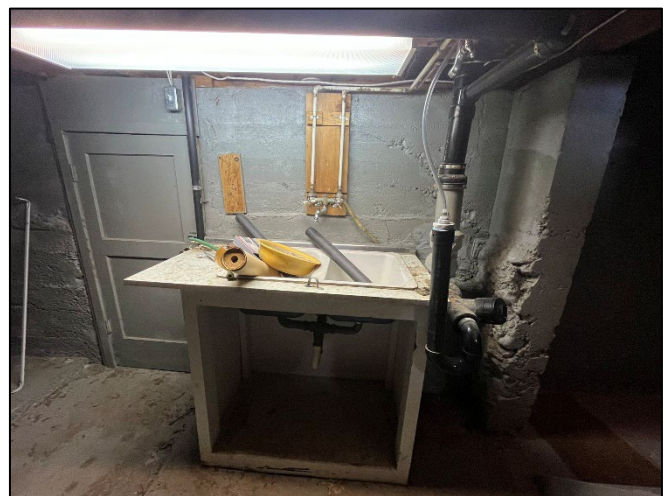
BASEMENT MECHANICS VIEW 2
