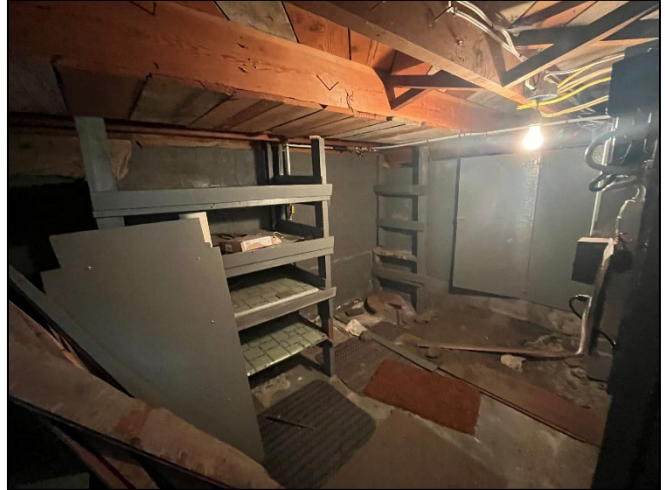
BASEMENT MECHANICS VIEW 4
